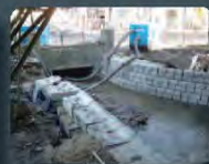
Erosion control of an underground stream. Listed building saved, wall took 3 men 17 days.
