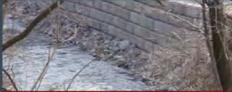
Engineered with toe-in to minimise erosion of the bank
