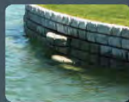
Jutting breaker blocks added to slow down current and prevent eddies forming
