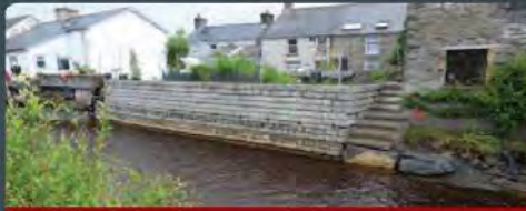
Homes protected from flooding in Tragaran - South Wales, Environment Agency specified
