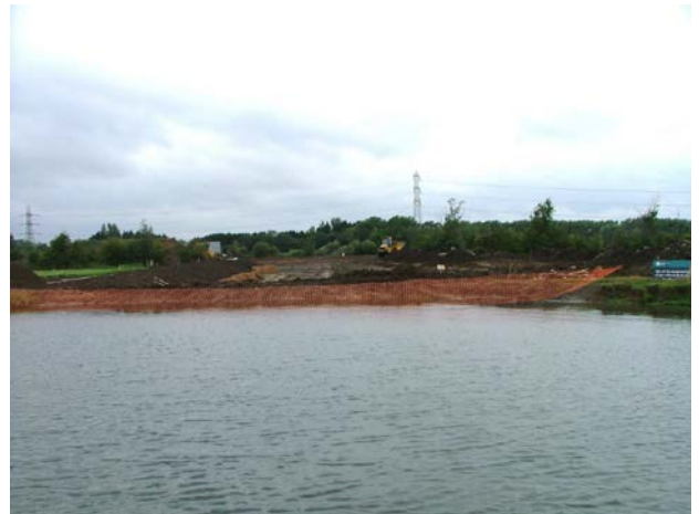
Construction works under way at the site of the new Jubilee Junction between the Wilts & Berks and the River Thames
