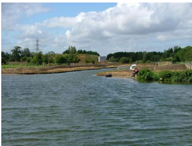
The completed Jubilee Junction, a month after the previous photo, showing the new section of the Wilts & Berks Canal
